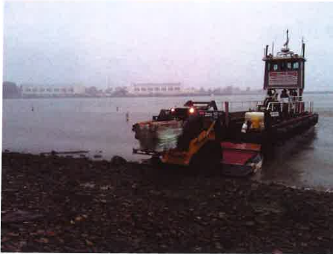
Equipment was brought in via barge because of the difficulty accessing Site YF3
