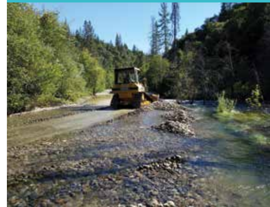
Below: A bulldozer contours a riffle from injected gravel at the "Below Dog Gulch" injection site at Clear Creek to help improve salmon spawning habitat.
