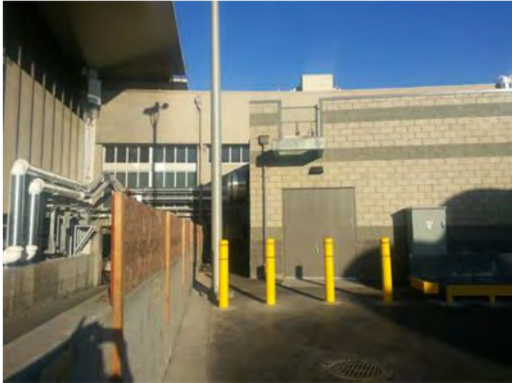
New Substation, Terminal 1 (M102)
