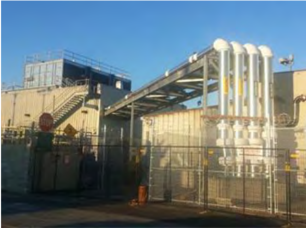
New Mechanical Building and Hydronics, T1CUP, Terminal 1 Area
