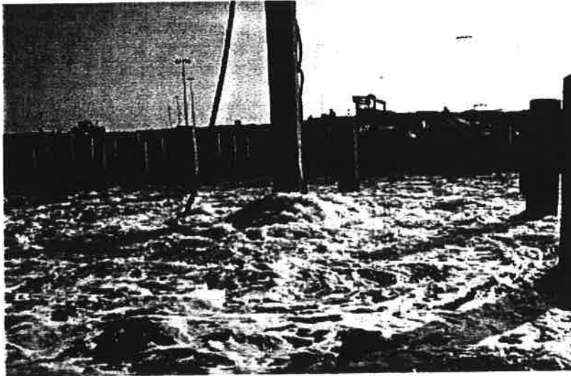
Figure 2. Air Bubble Curtain Attenuation System in Operation.
